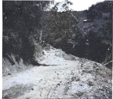
Widening road for trucks preparatory to hauling in mill parts and supplies.
