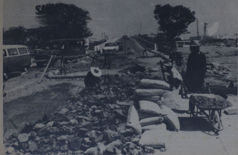
Manila construction project: beating the deadline before the onset of the rainy season.
